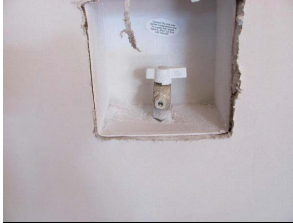
No water hammer arrestors
