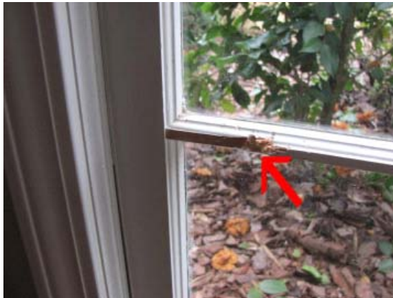
One of the windows is damaged near the bottom. Repair or replacement is needed.
